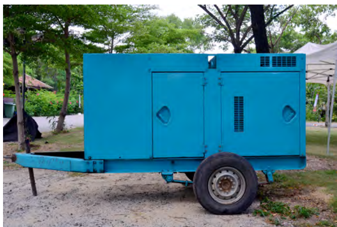
Abb. 5.17 Biogasgeneratoren Photo: Adobe Stock | tuayai
